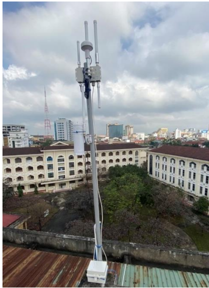
Fig. 11. RAK2490 Gateway installed at University of Sciences, Hue University
